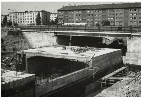
Figure 6 Construction of Metro Line C, view toward Olbrachtova Street, 1971. Source: 40 let DBK, 40let.dbkpraha.cz
